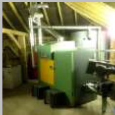
200kW Biomass Boiler
