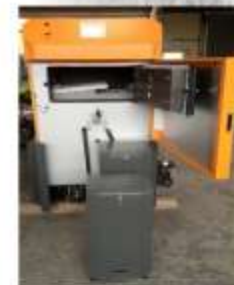
199kW System Kurri boiler
